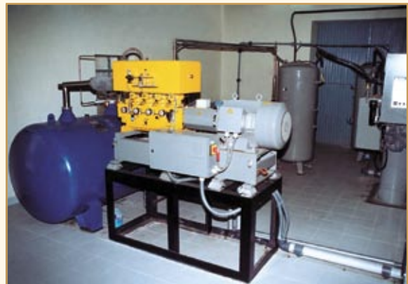
STIRLIN - 4 Liquid nitrogen Plant (capacity 44 litre/hour)
