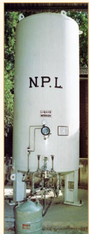
Liquid nitrogen storage dewar of 6000 litre capacity
